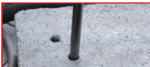
Dust buildup using our CLEAN EXPERT
